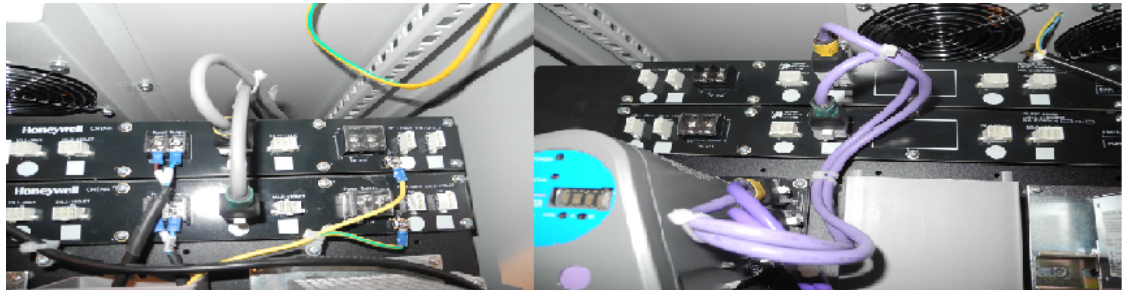
Figure 3: Cabling for the power distribution subsystem
